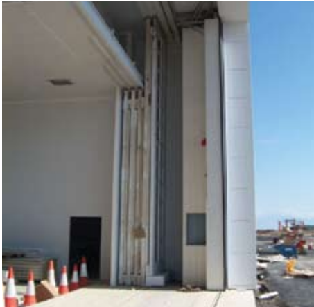
The doors are sealed with flexible seals along the top, bottom and sides to prevent loss of air or the introduction of contaminants.
