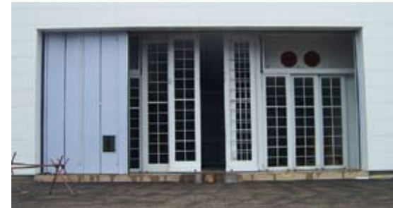
In a pressurized paint spray booth, solid bottom rolling doors are placed in front of the filter doors to create a plenum space enclosed by the two doors.
